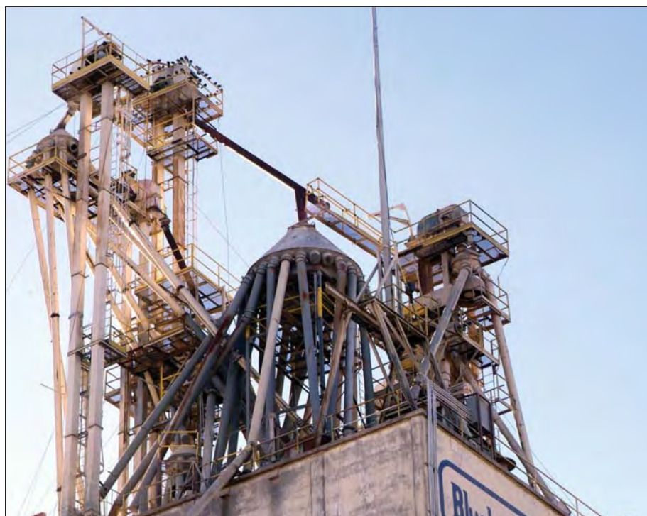
Upgrades on the roof of the feed mill include four new Hayes & Stolz electric distributors and a lot of stainless steel spouting.
