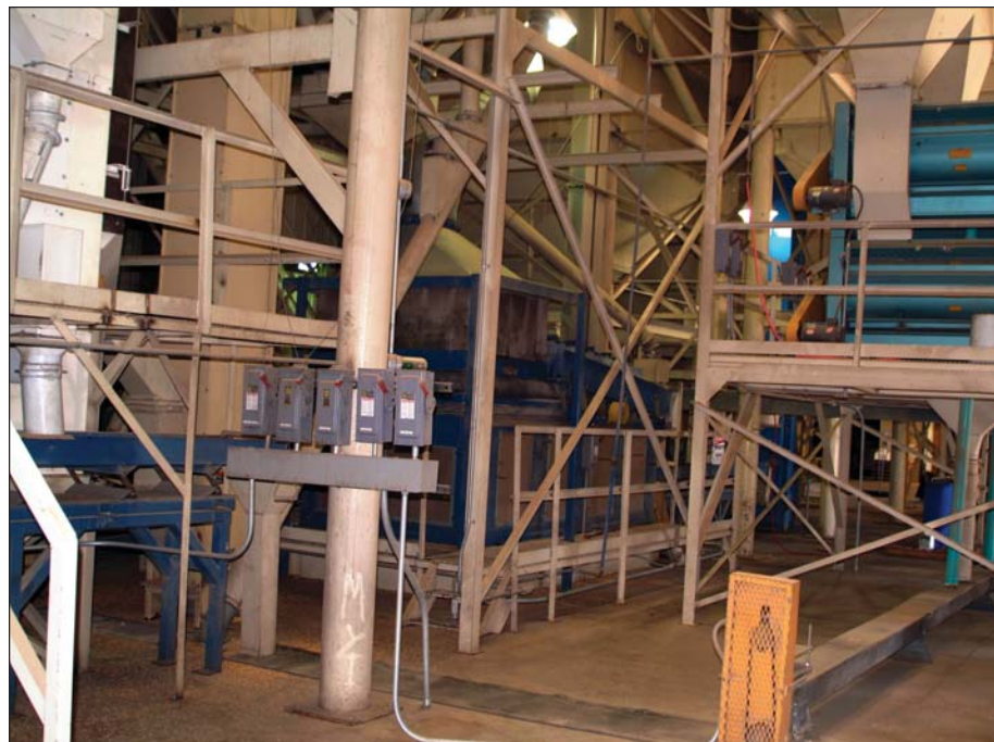
Most of the conditioning equipment is on ground level or a low-level mezzanine.
